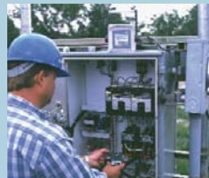
Isco 4501 Pump Station Monitor
